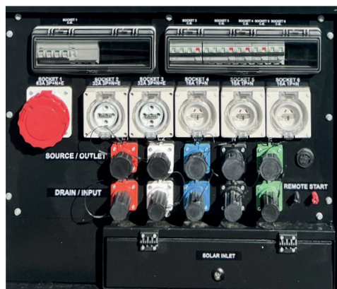
Example of electrical panel
